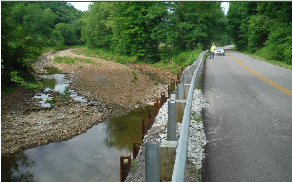
Slope/shoulder stability issues adjacent to the roadway near Eddie Stamm Farm at Indian Creek.
