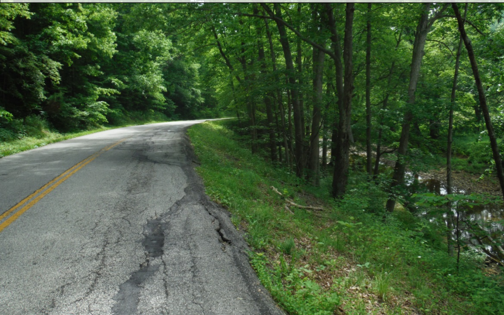
Slope/shoulder stability issues adjacent to the roadway at Indian Creek. 5/29/2015
