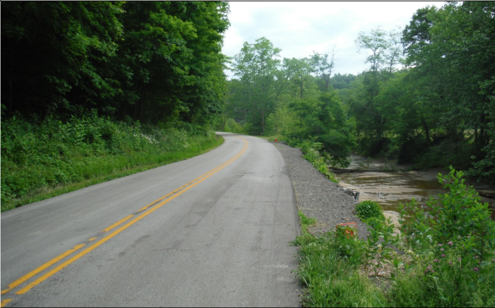
Slope/shoulder stability issues adjacent to the roadway at Mike Thomas Place at Indian Creek.
