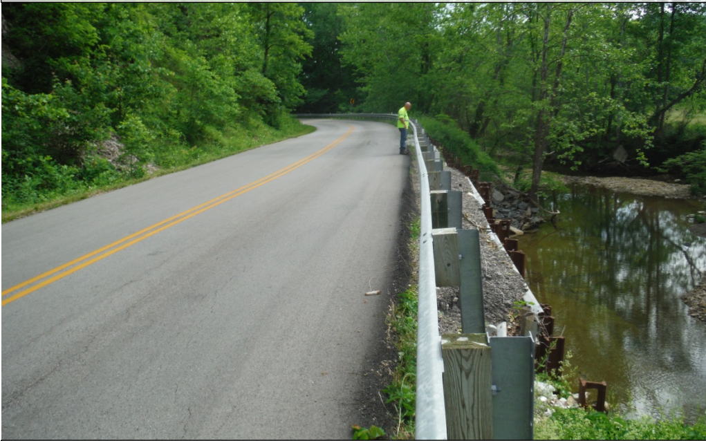
Slope/shoulder stability issues adjacent to the roadway near Eddie Stamm Farm at Indian Creek. 5/29/2015
